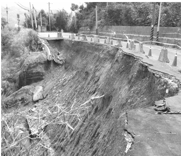
Fig. 5 RSS collapsed during an attack of typhoon
