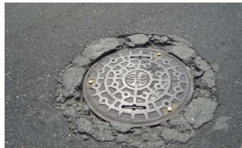
Figure 2 deteriorated pavement surrounding manholes
